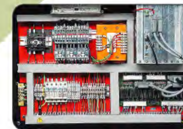
Compact electric box with circuit board.
